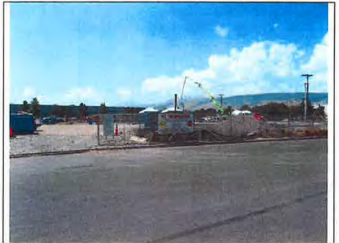
34. View of adjacent property to south (west portion) across Innovation Drive, active construction site.
