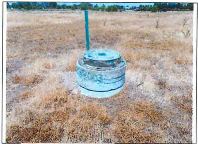
26. View northwest of municipal sanitary sewer access in east-central portion of subject property.
