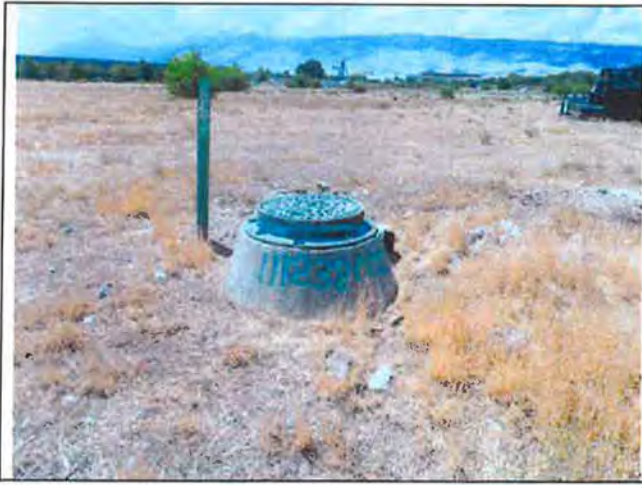
25. View south of municipal sanitary sewer access in northeast portion of subject property.
